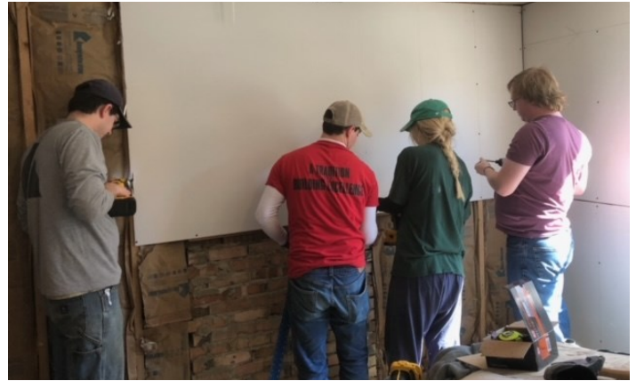
Four BCM students help hang drywall in a house in Jenkins, KY.
