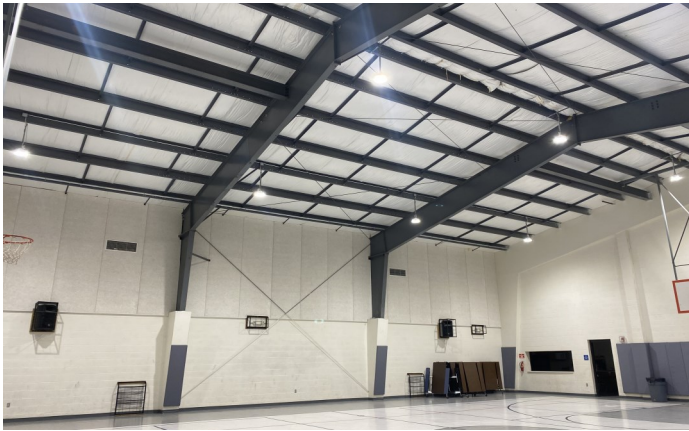
New LED lighting in the Greenlee Activity Center.
