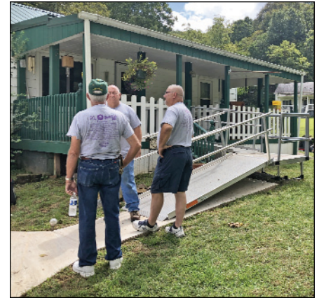
A wheelchair ramp is installed for a member of Leon Baptist Church.
